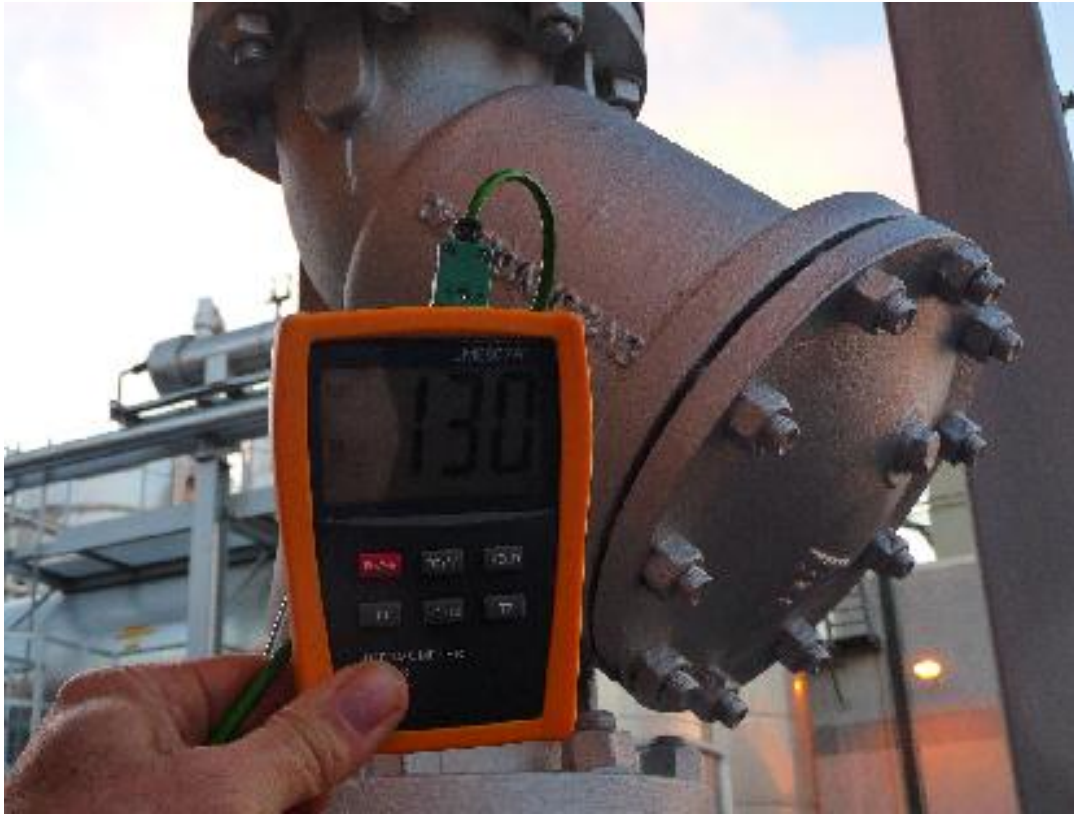
Uninsulated – primed pipework- 130°C
