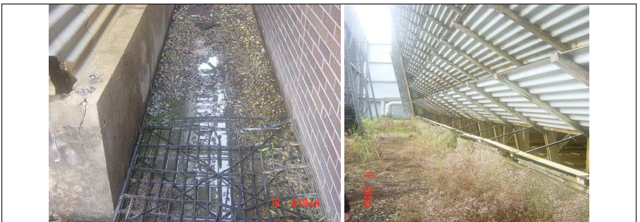
The pictures show the accumulation of water from a leaky basin.
